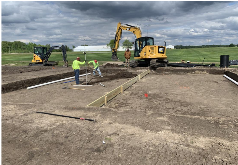
Figure 2. Workers leveling the subgrade of a Capillary Hydroponic System green at the Capillary Hydroponic System and Variable Depth Rootzone research site at Michigan State University. The wooden board splits the green into two equal halves and will be covered by an impermeable liner. The control basin seen in the background to the right of the excavator will be installed adjacent to the green and house components that will move water inside the cavity back and forth between the two equal sections.
