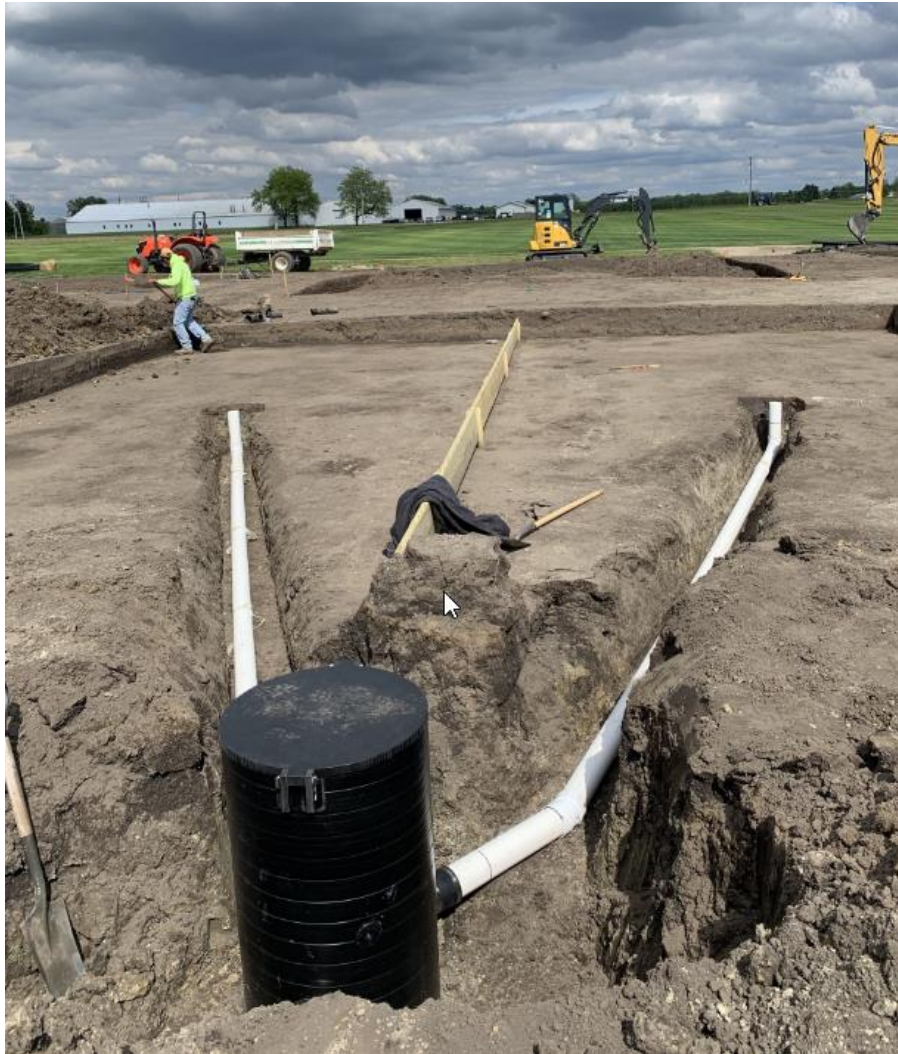
Figure 4. Control basin (foreground) installed adjacent to a Capillary Hydroponic System green at the Capillary Hydroponic System and Variable Depth Rootzone research site at Michigan State University. Two inlet pipes installed below the subgrade and extend from the bottom of the basin to the surface at the center of each half of the green's cavity allow for water to flow from the cavity to the control basin.
