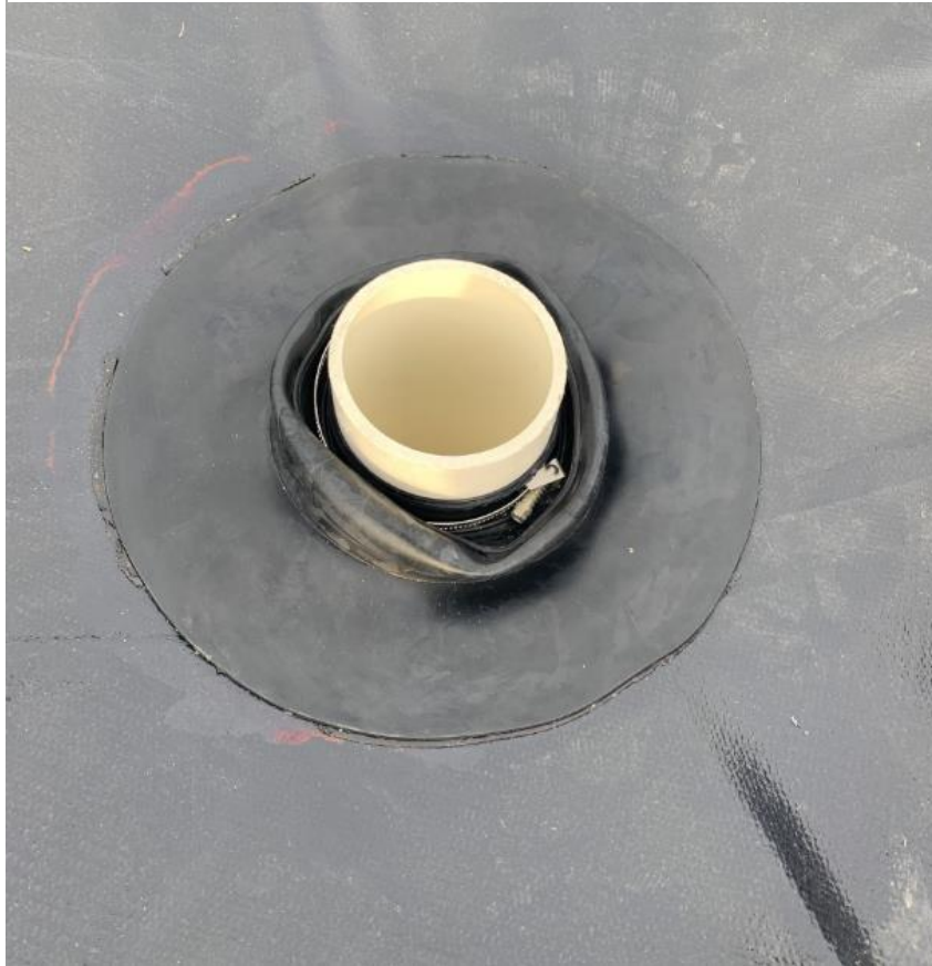
Figure 6. A rubber gasket adhered to the liner that lines the cavity of the Capillary Hydroponic System at the Capillary Hydroponic System and Variable Depth Rootzone research site at Michigan State University. The gasket is hose clamped around the inlet pipes to prevent water loss in the Capillary hydroponic system.
