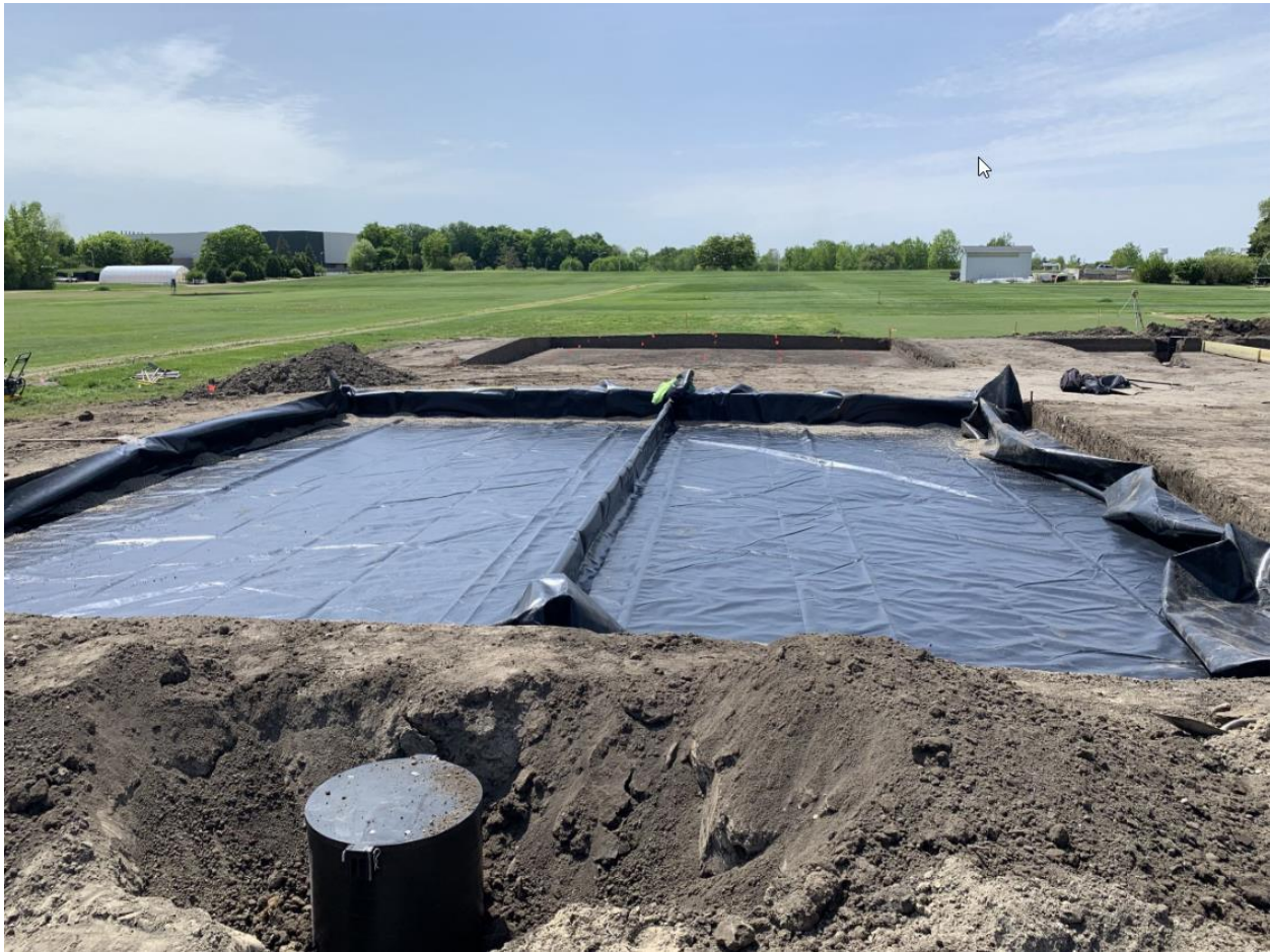
Figure 5. A waterproof liner installed to line the Capillary Hydroponic System green cavity at the Capillary Hydroponic System and Variable Depth Rootzone research site at Michigan State University. The liner creates a closed system and allows for the cavity to hold water.
