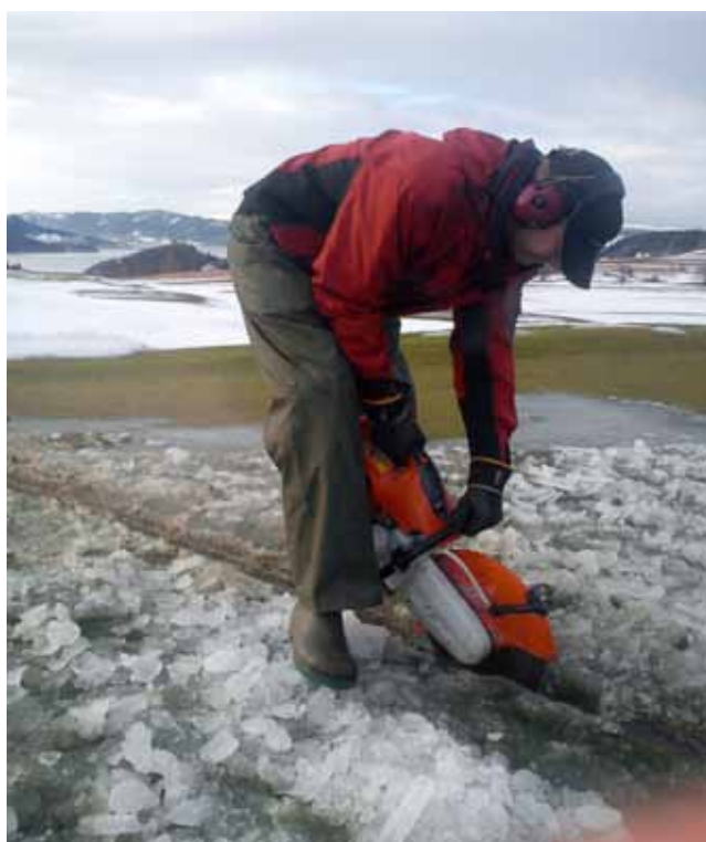
An asphalt cutter used to restore a drain out of the green. Photo: Ole Albert Kjøsnes, Byneset golf.
